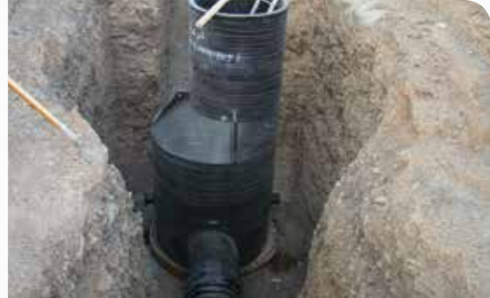
NIC HDPE Corrugated Pipes for Sanitary / Sewerage water, connecting to HDPE Manholes, project in Oman
